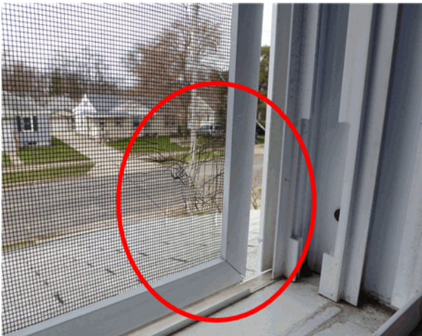
Bedroom 1 screen torn
