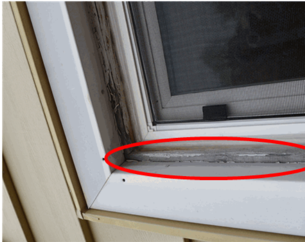
Exterior blind stop peeling paint on vinyl replacement windows.
