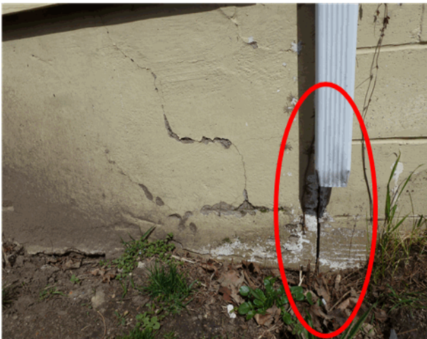
Downspout needs to be diverted away from the structure
