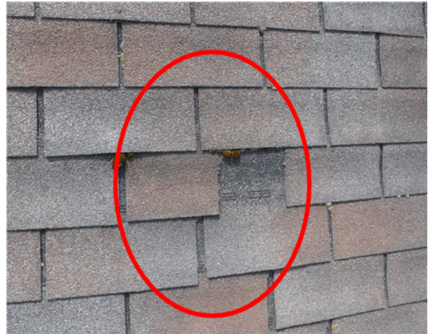
Missing shingle of south side garage roof.
