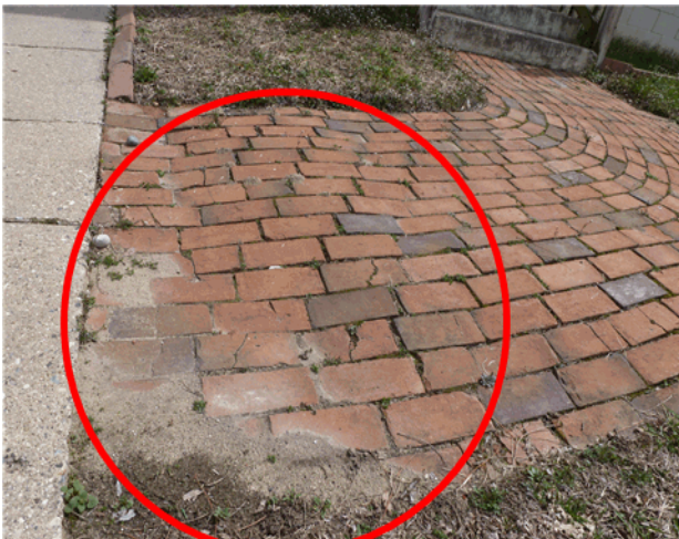
Front entry brick sidewalk settling possible trip hazard.
