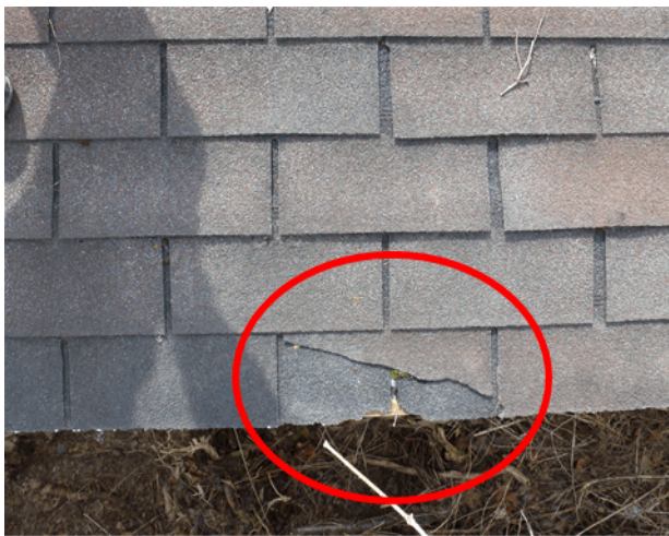
Damage on the eave of the north side garage roof.
