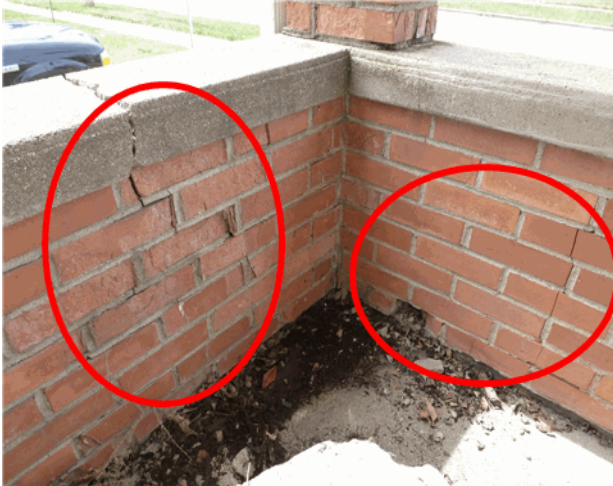
Front porch brick settling and deteriorating.
