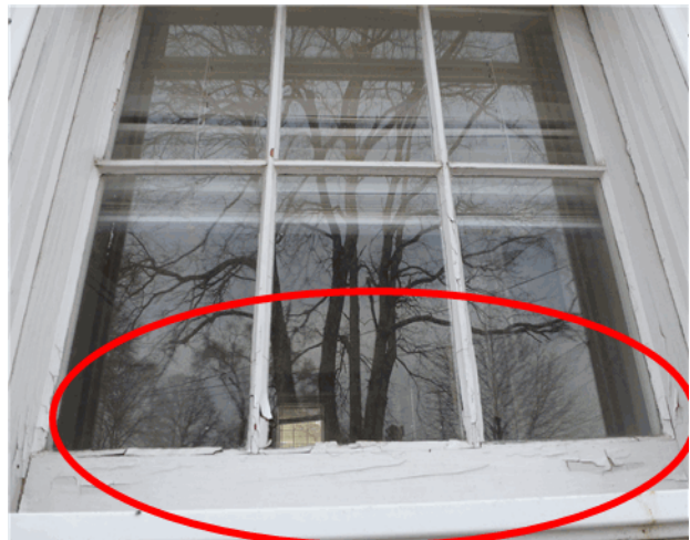
Exterior window glazing deteriorated and peeling paint
