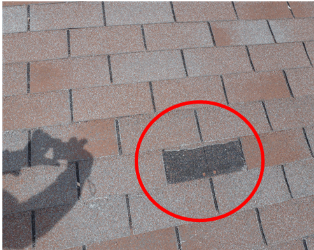
Missing shingles on south side of garage roof.
