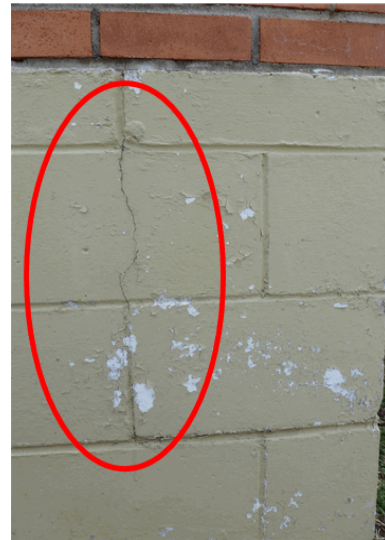
Minor cracking at north corner of front porch.
