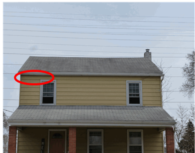
Siding needs repaired to prevent insects and weather from entering building.
