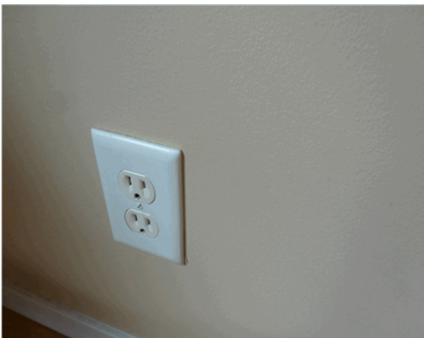
Masterbed electrical receptacle loose.
