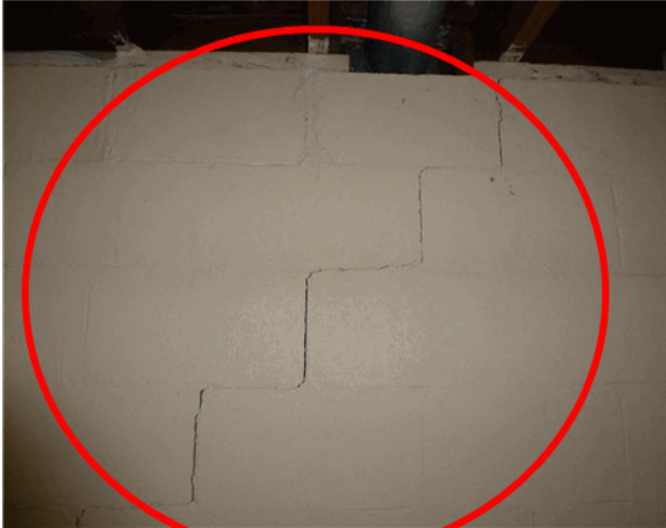
Laundry room exterior wall cracks.
