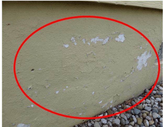
Loose paint at exterior basement walls.
