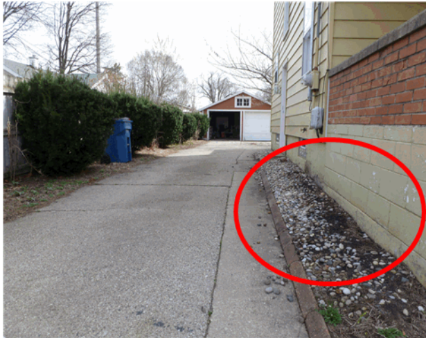
Weather exterior basement wall have loose paint and mortar.
