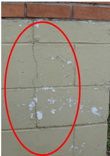
Minor cracks and peeling paint on north side foundation wall.
