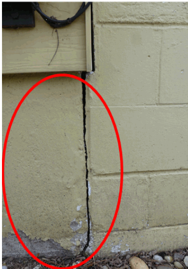
Porch north side minor cracking.
