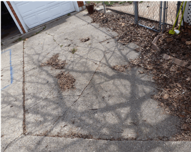
Minor cracking and settling in driveway.
