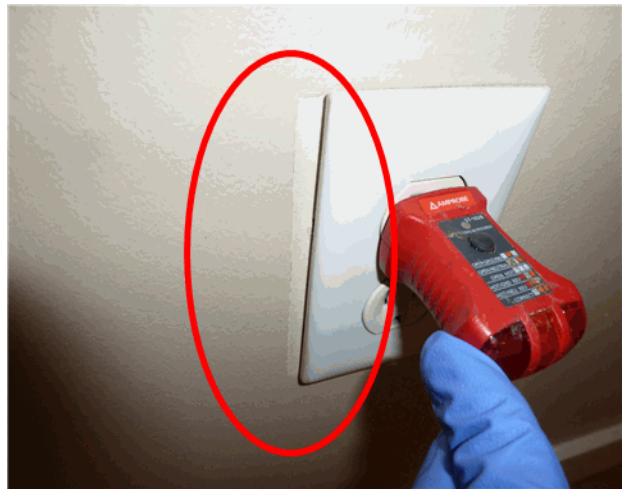
Bedroom 2 electrical receptacle loose
