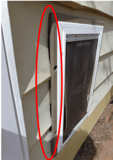
Pet door not sealed insects and elements can enter the building.
