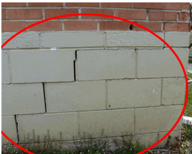
Front SW corner major crack and settling.
