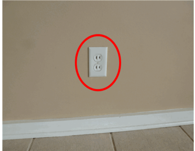
Sunroom electrical receptacles do not have a ground.
