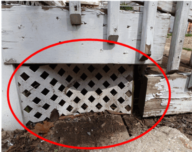
Bottom lattis damaged
