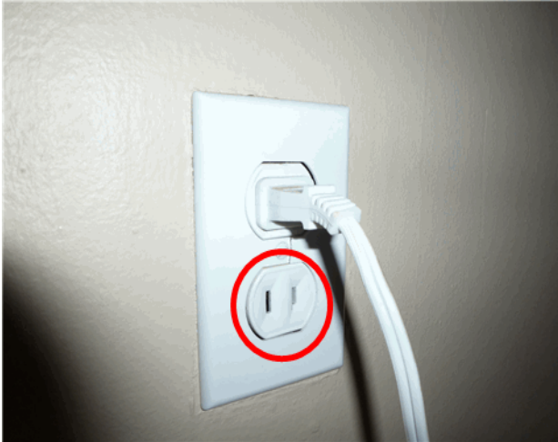
No ground on living room electrical outlets
