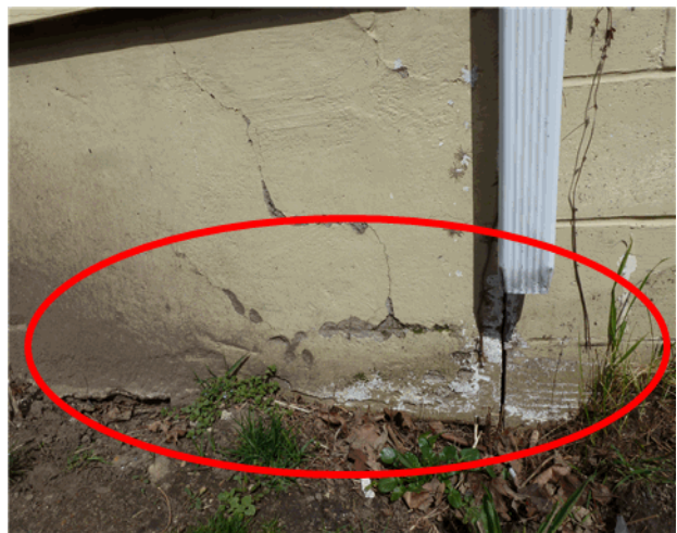
South side exterior basement wall cracked mortar and peeling paint.
