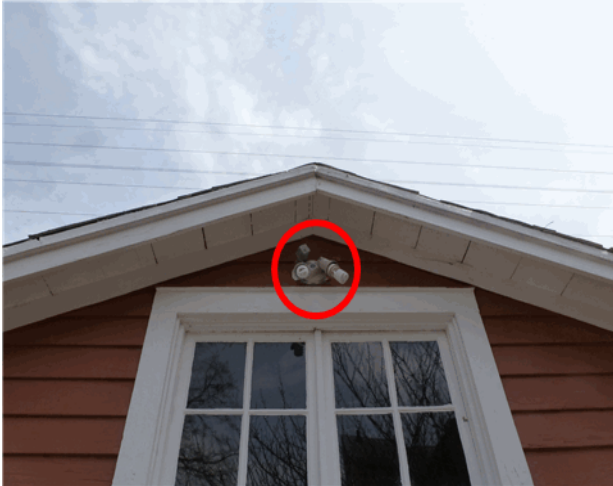
Garage light bulbs not exterior rated.
