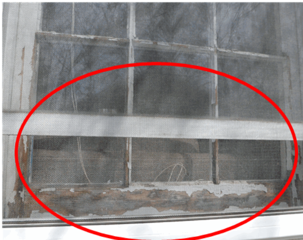
Peeling paint observed in every window.
