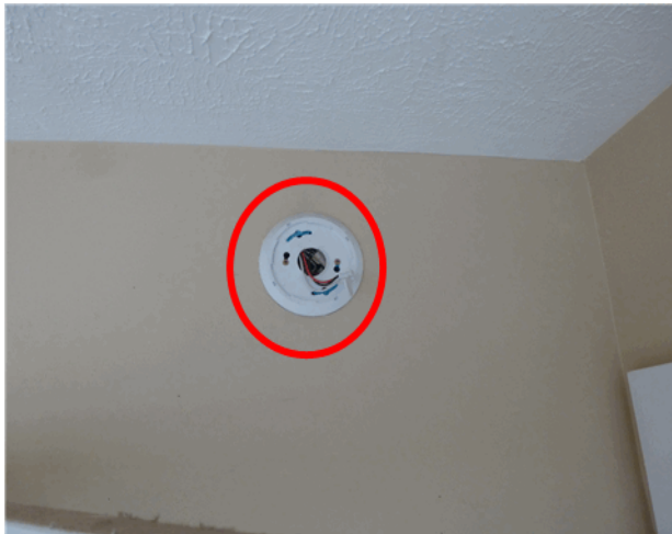
Rear Sunroom smoke detector missing.
