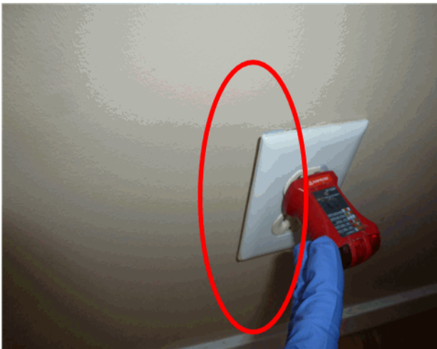
Bedroom 1 outlet loose.
