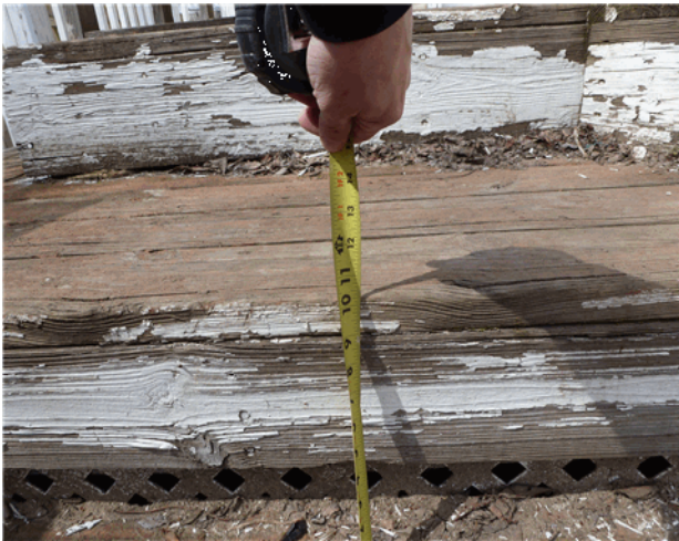
Top Step height 10 1/4" is considered a trip hazard
