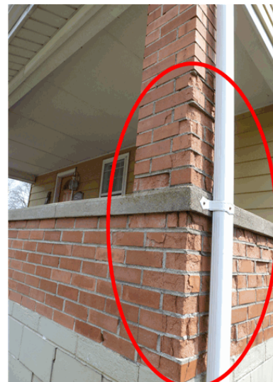
Settlement has occurred please contact structural engineer to determine structural integrity.
