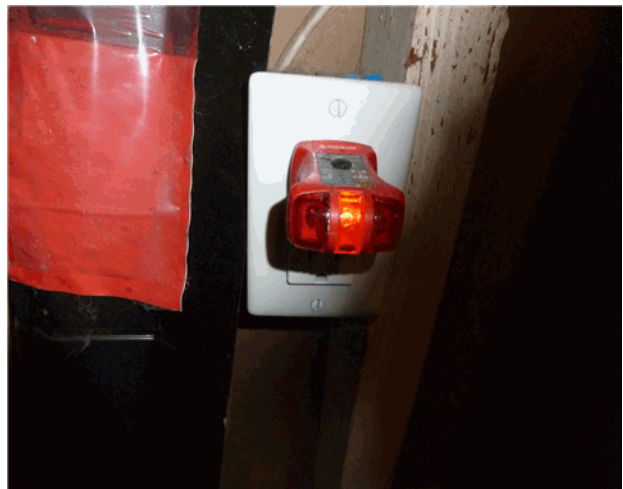
Basement laundry room GFIC failed. Outlet has an open ground.
