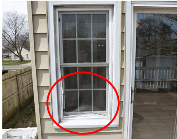
Damaged Screen Rear elevation
